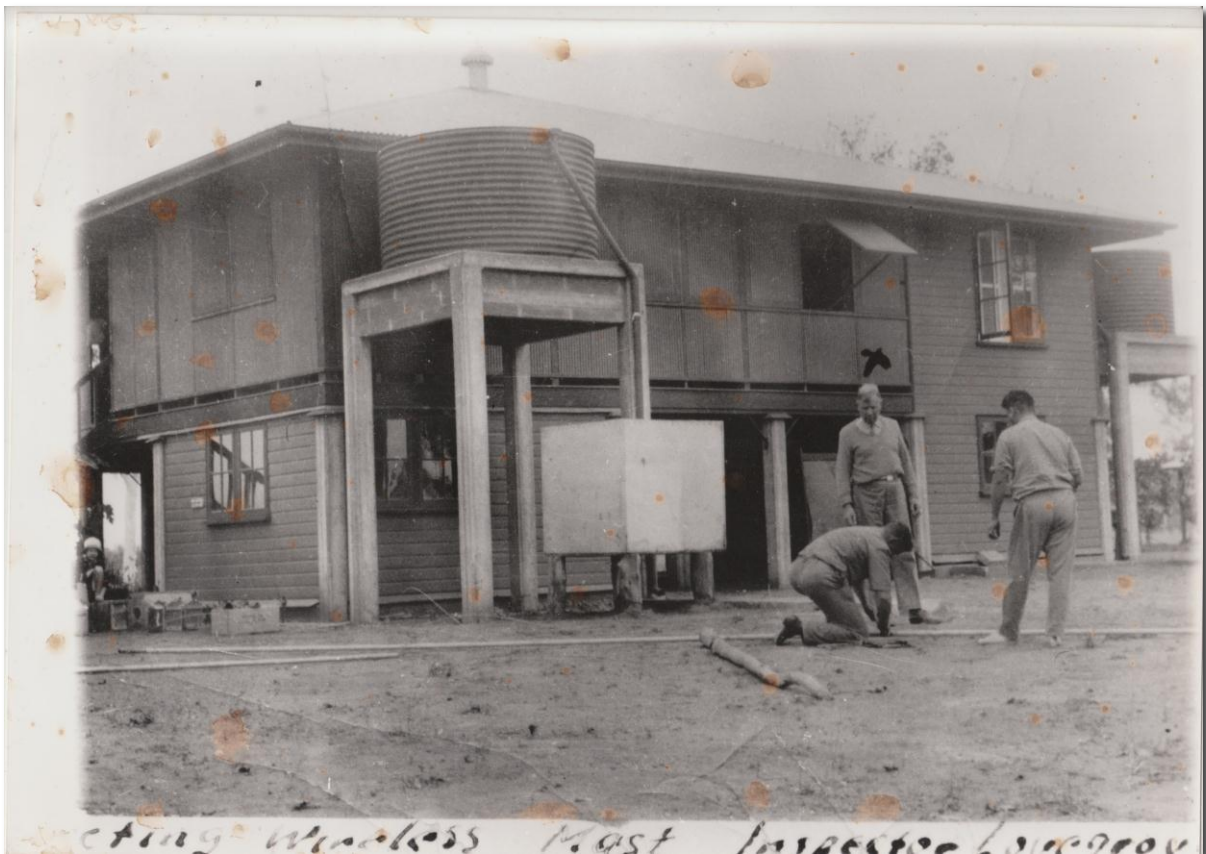
Preparation for the erection of the wireless mast at Roper River Police Station. From left to right, Lew Curnow, Inspector Lovegrove with cross marked above his head, and Charlie On. Inspector John Creed Lovegrove’s son is featured in a story later in this edition.
