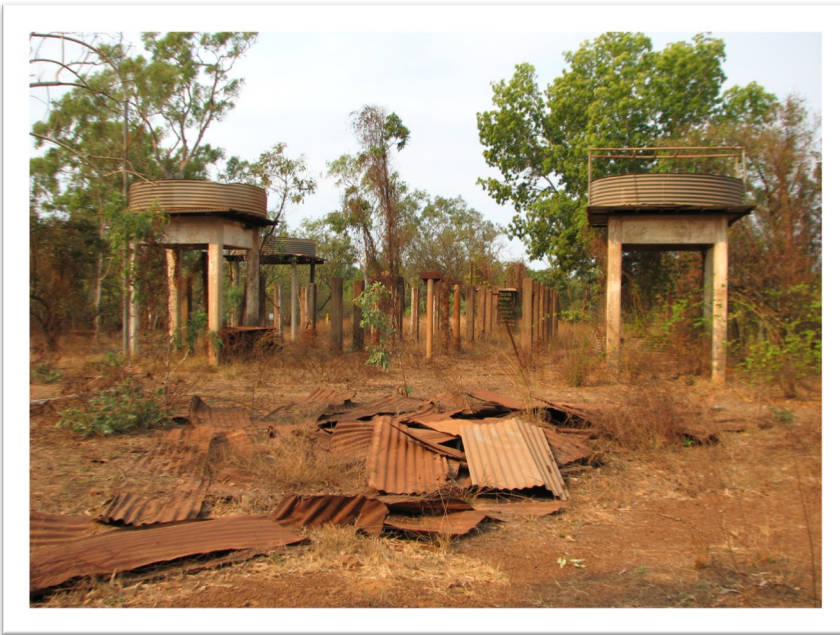
Roper Bar Police Station—after the fire
